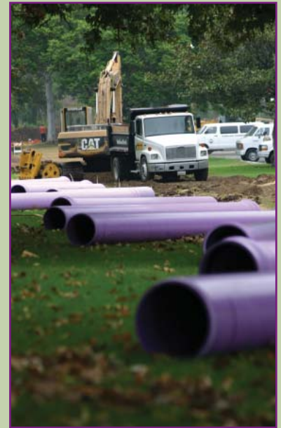
Construction crews worked on a reclaimed water line project near the north end of the campus. Reclaimed water is piped in from the nearby Camrosa Water Treatment Plant to irrigate University landscapes, as part of the University's commitment to a green campus.
