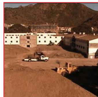
John Spoor Broome Library construction as viewed from the Library Web Cam.
