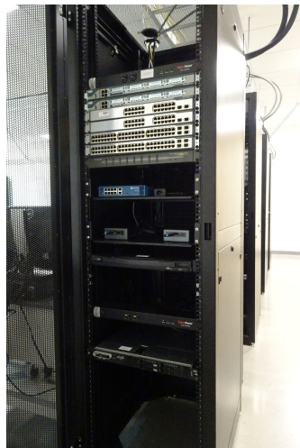
A view of one of the 8 rack cabinets in SIE 1131 filled with the equipment purchased from the grant.
