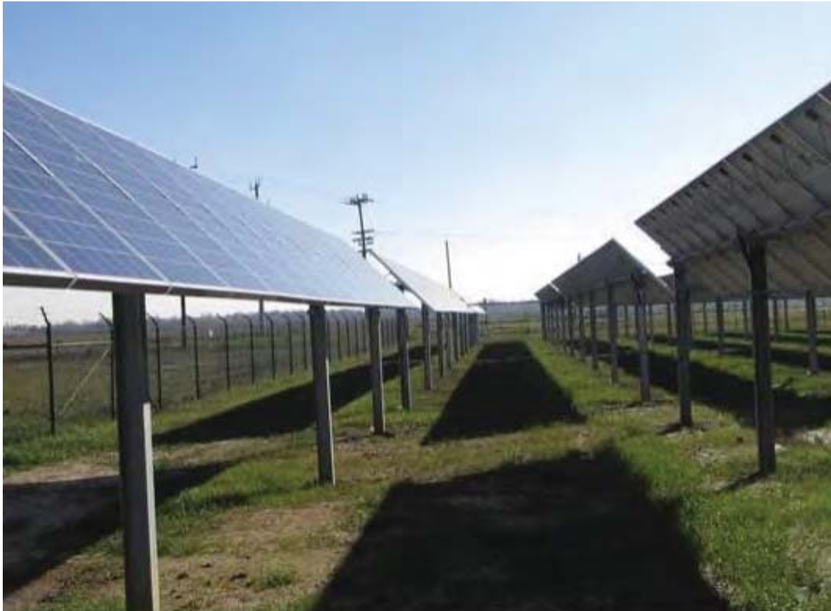
Figure 9 Example of Solar PV Array Over Open Ground
