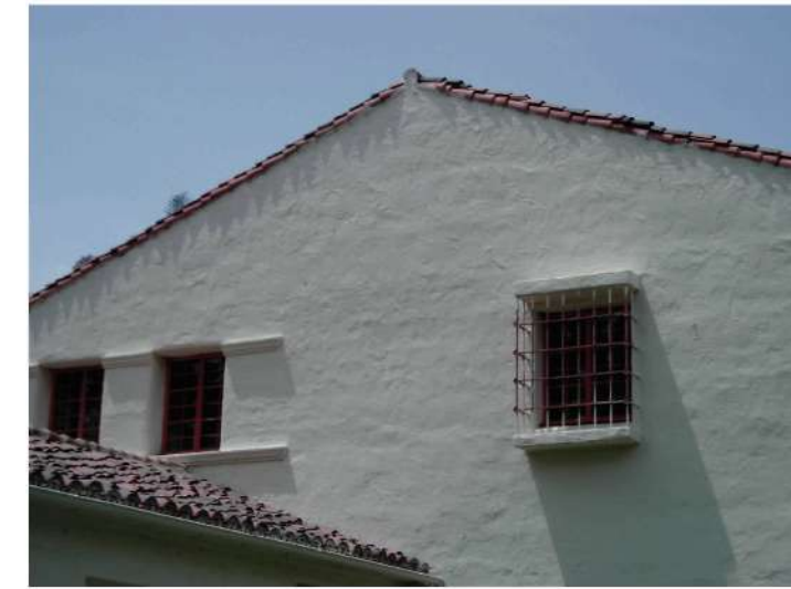
Gable Ends (Note: Tight or No barge)
