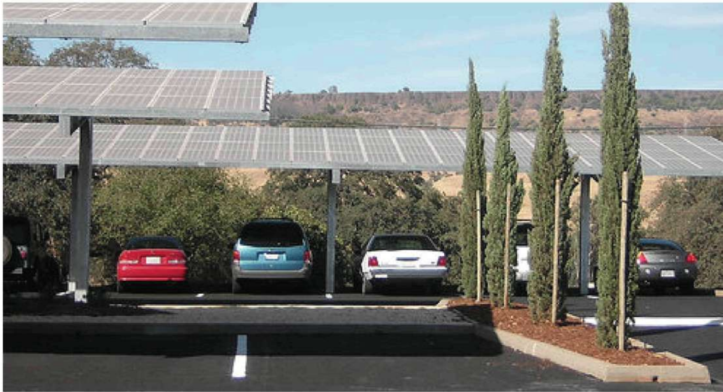
Solar: Photo Voltaic Panels
