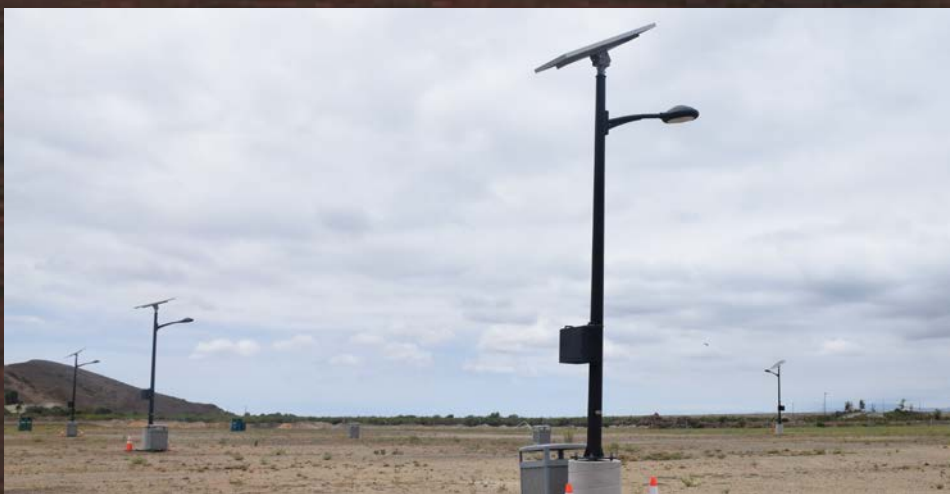
Pictured Above: Solar parking lot lights
